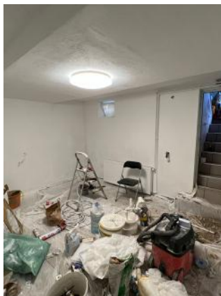
Walls have been painted. Floor has been tiled! Not much more to do!
